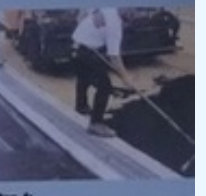
Step 4: Add paving surface flush to the top of trench grate, to move the water flow across pavement into the trench.
